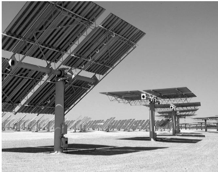
Figure 13: Detail of a heliostat [4]
