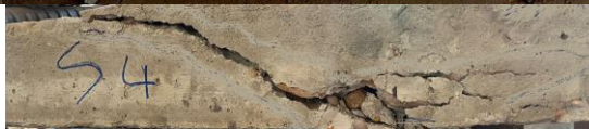
(c): Pattern of cracks of the slab strengthened with steel plate at the bottom surface.
