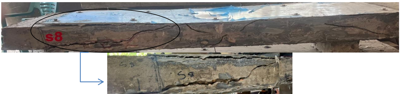
(g): Pattern of cracks of the slab strengthened with Aluminum-CFRP at the top and bottom surfaces. Figure 7: Patterns of cracks of the sandwich reinforced concrete slabs.
