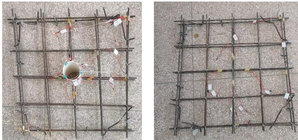
(a) Reinforcement cage for SOBC specimens (b) Reinforcement cage for SOAC specimens Figure 4: Binding steel reinforcement cage for specimen
