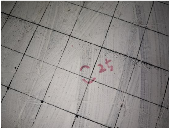
Figure 2.19 Top crack of concrete slab at right end (Grade 10)
