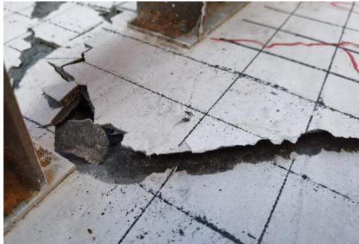
Fig. 3.20 Peeling of concrete slab bottom
