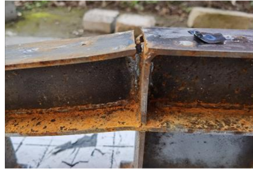
Figure 2.31 Fracture of the lower chord (inverted)
