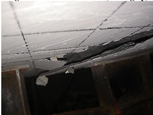
FIG. 2.27 Serious peeling of concrete slab bottom (Grade 17)
