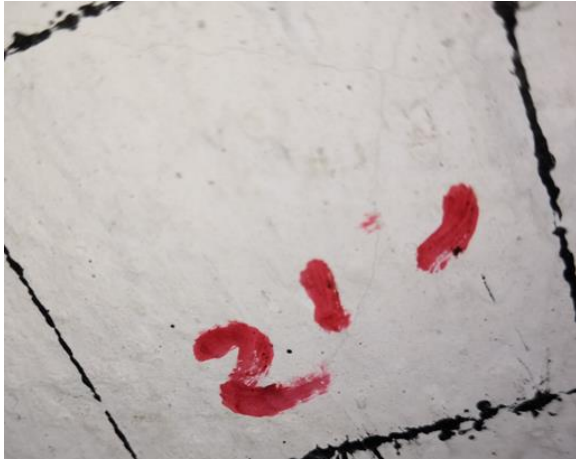
Figure 2.14 Crack No. 2 (Grade 7)
