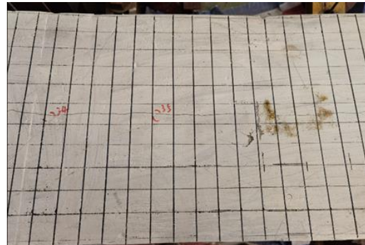
FIG. 2.33 Cracks in the top of the plate along the long direction of the beam
