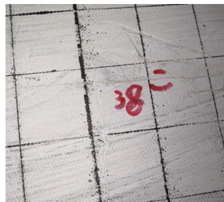
Figure 2.22 Longitudinal cracks on top of concrete slab (Grade 15)
