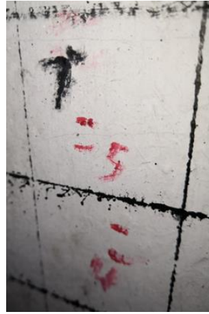
Figure 2.15 Cracks No. 4, 5 and 7 (Grade 7)
