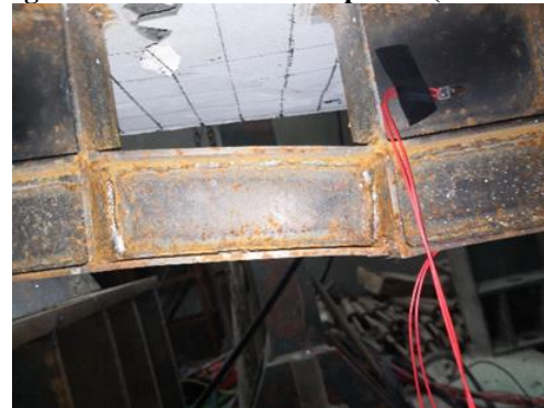
FIG. 2.28 Expansion and severe deformation of chord fracture (Grade 17)
