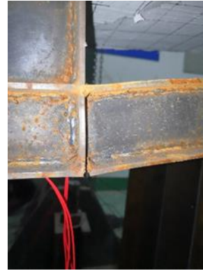
Figure 2.24 Chord fracture (side view)
