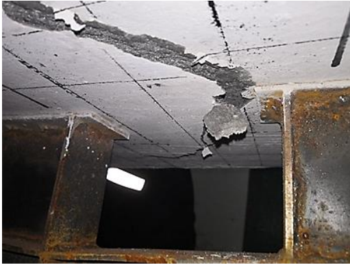
Figure 2.23 Peeling of concrete (Grade 16)
