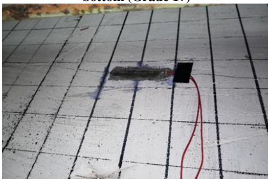
Figure 2.29 Longitudinal penetration of cracks in the top of concrete slab
