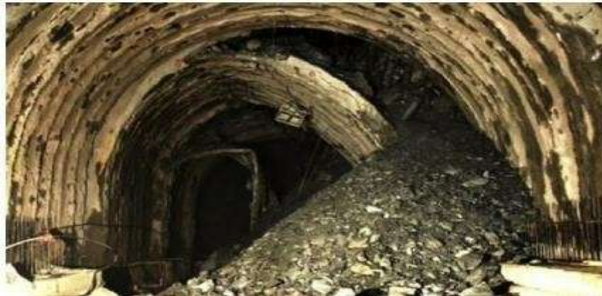
Figure 1: Deterioration in the tunnel towards extending
