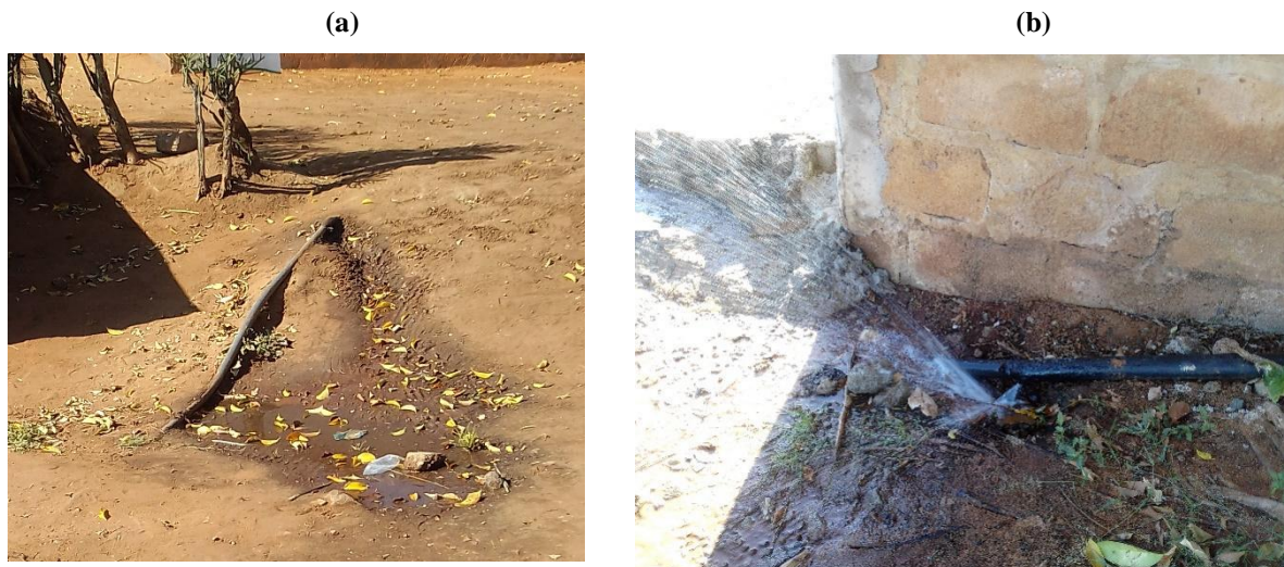
Figure 5.7 pictures of water leakages (Source: Field Observations)
