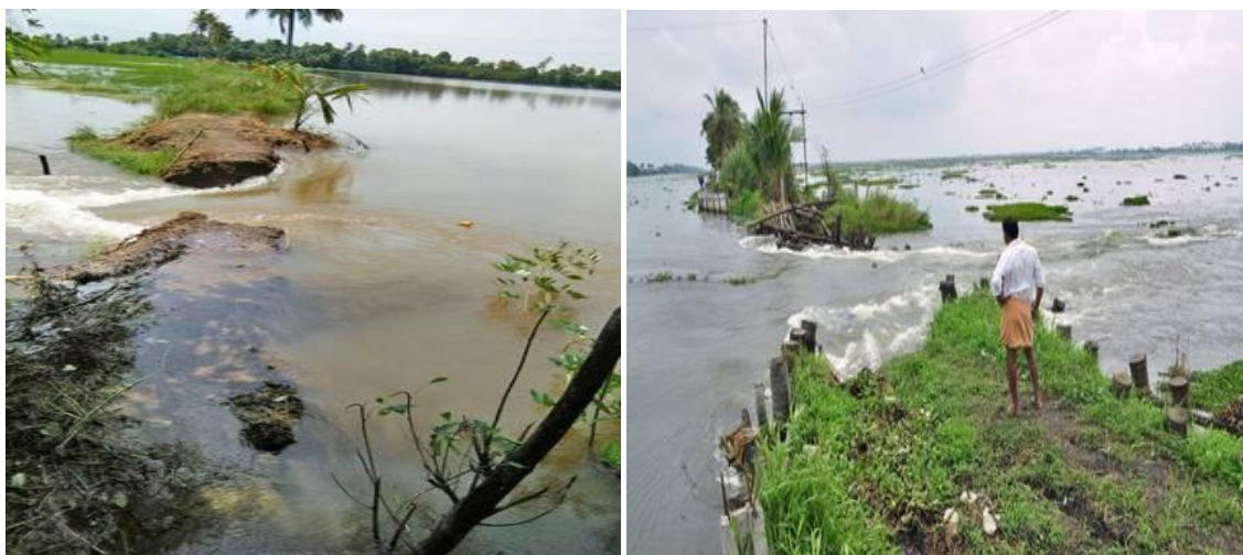
Figure 3. Bund breach during flood
