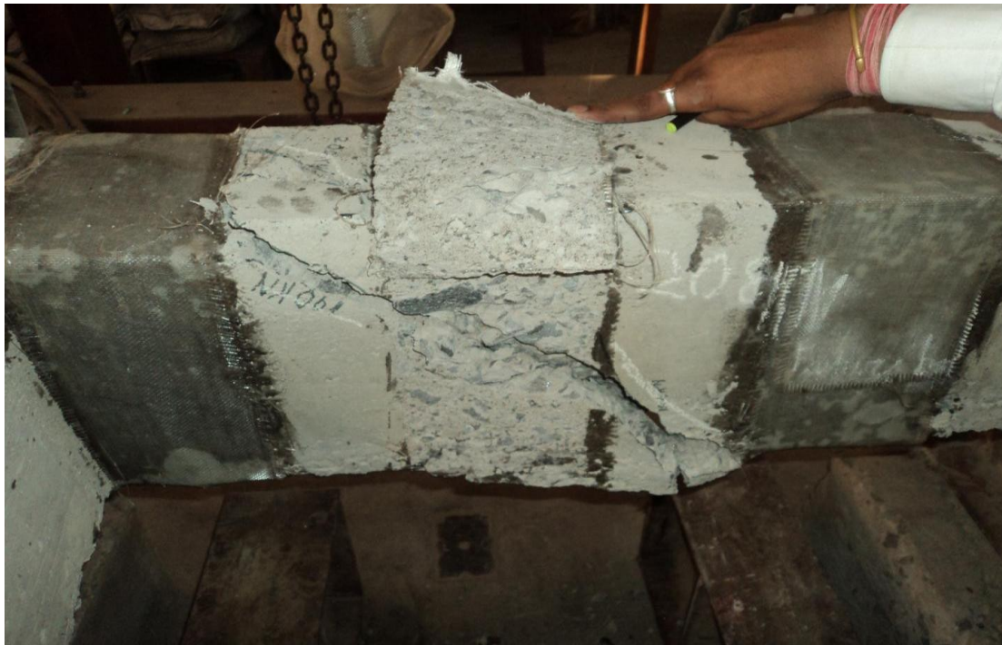
Figure 14 shows the failure pattern of the retrofitted beam, when the GFRP sheet was removed.
