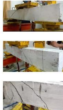
Fig-1 Crack patterns on Control Beam after Flexural test
