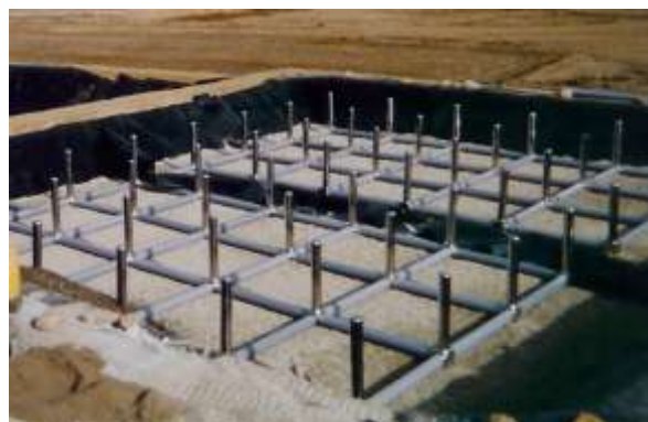
Figure 2: The natural air draft system installed inside the aerobic tank of the constructed wetland
